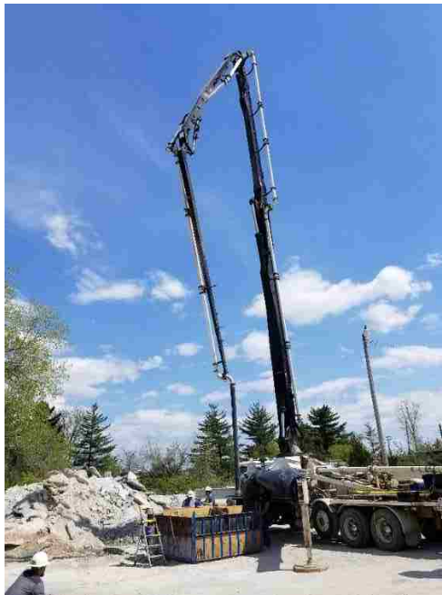
Figure 4-4 Pump on "A" configuration.
