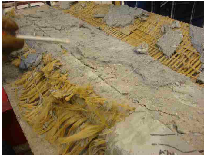
Figure 10. Distribution of concrete cracks beneath the FRCM composite for beam N-P-4-C-2.
