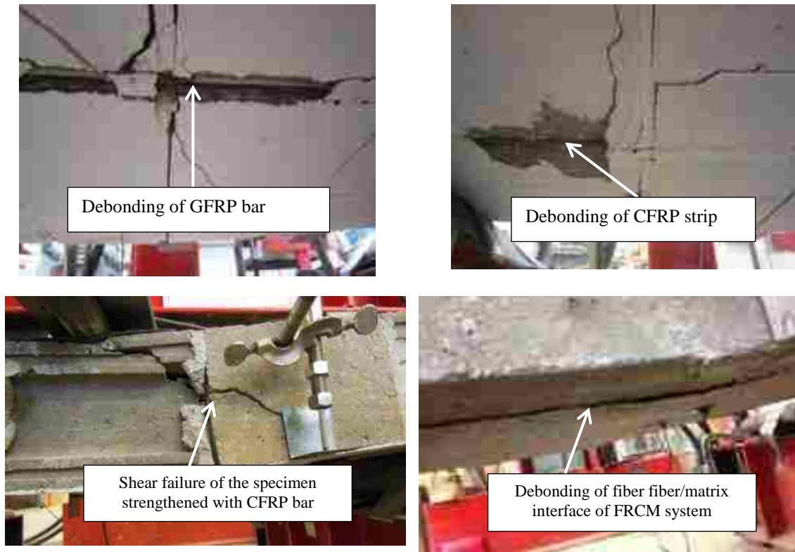
Figure 13. Observed modes of failure
