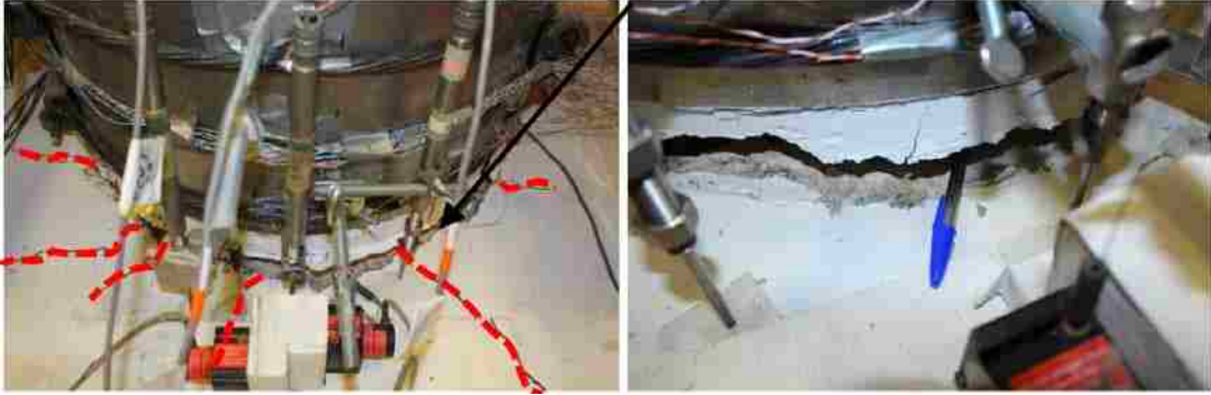
FIGURE 8 Concrete cracks associated with stress transfer through dowel bars at the column-footing connection
