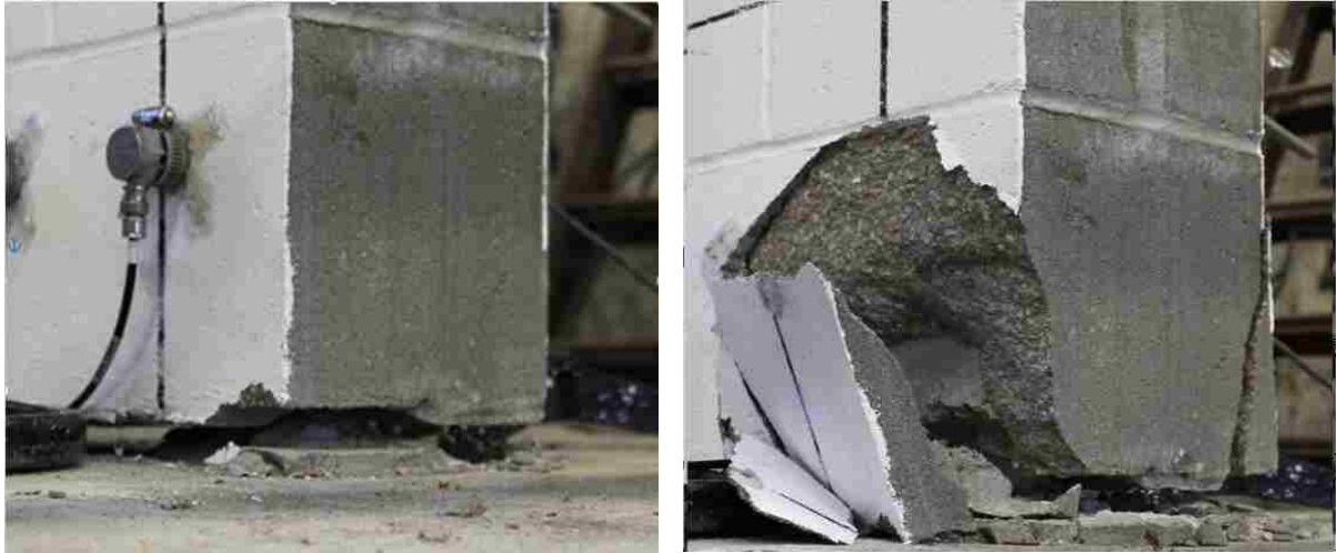
(a) Separation at the Bed Joint
