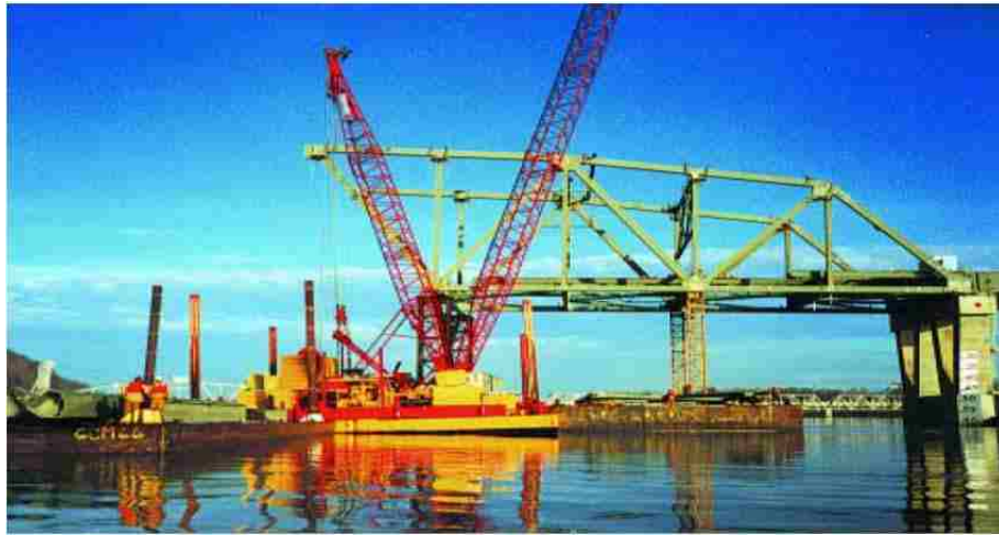
Figure 9.3. Single Span Construction using Shoring in the River. Image from Niemietz and Bauer (1999)
