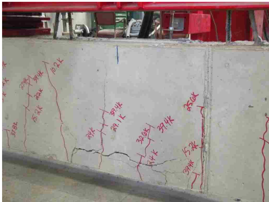
Figure 5.12 – Failed control specimen with confinement
