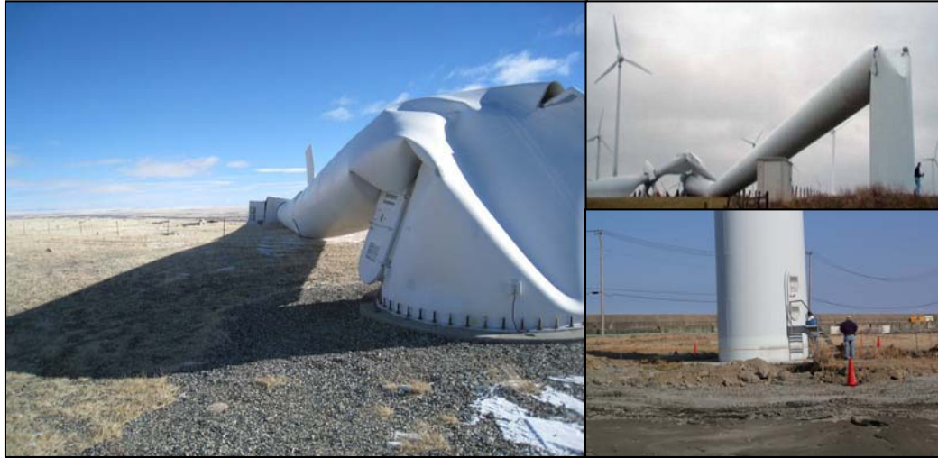
Figure 1.3 Turbine failure due to earthquake loading in Japan and New Zealand
