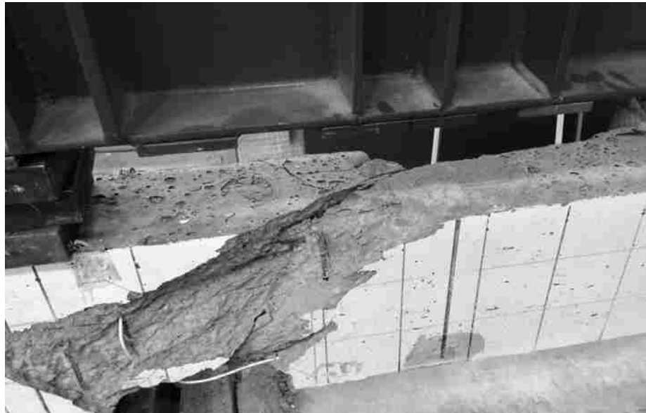
Fig. 12. Failure mode of GL6-2
