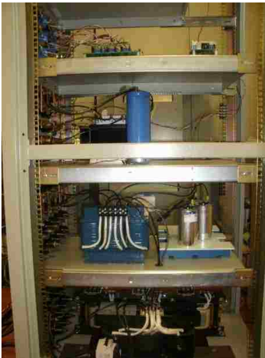
Fig. 7 (a) Sensor, Interface and DSP boards (1 st ), Dc-link capacitor and Inverter (2 nd ), LC filter (3 rd ), Isolation Transformer (4 th )
