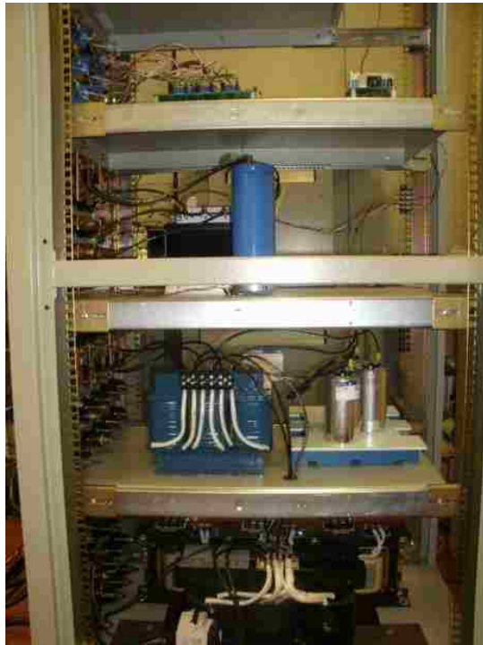
Fig. 8 (a) Sensor, Interface and DSP boards (1st), Dc-link capacitor and Inverter (2nd), LC filter (3rd), Isolation Transformer (4th)
