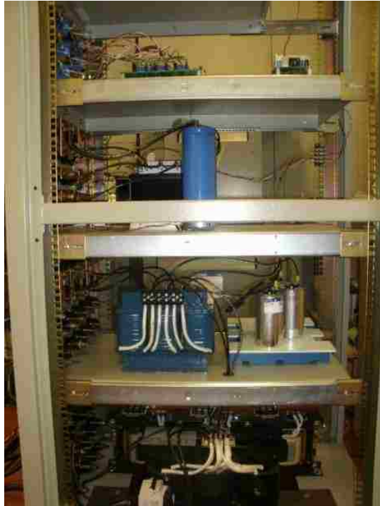
Fig. 8 (a) Sensor, Interface and DSP boards (1 st ), Dc-link capacitor and Inverter (2 nd ), LC filter (3 rd ), Isolation Transformer (4 th )
