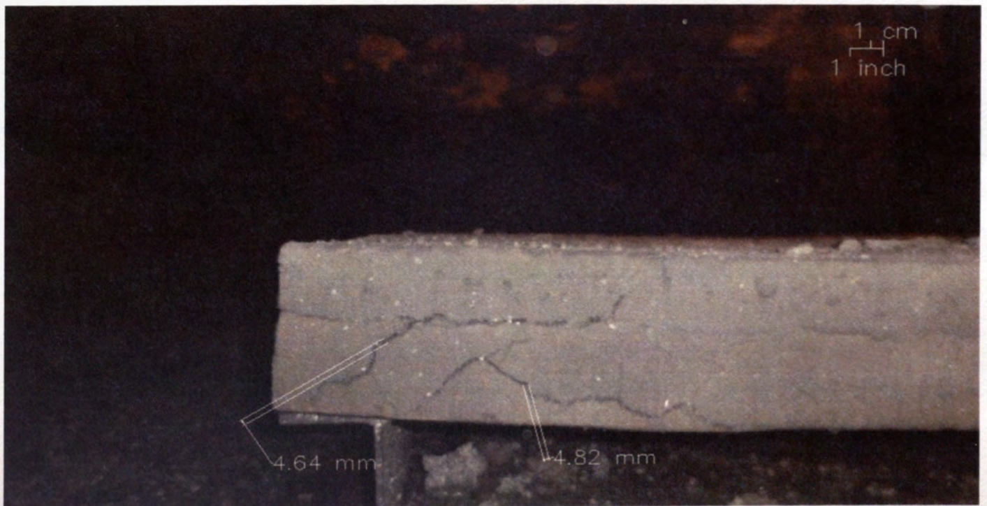
Figure E.15 – Shear Cracks in the Front Face of H-B, 2 nd Event
