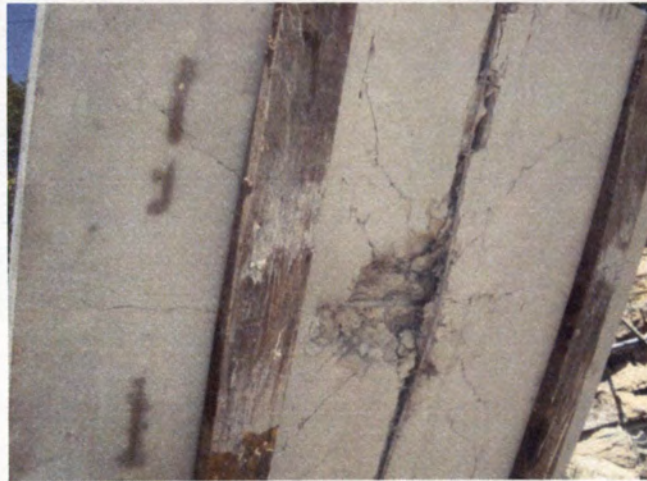
(c) Flexural Crack and Spalling on Tension Face
