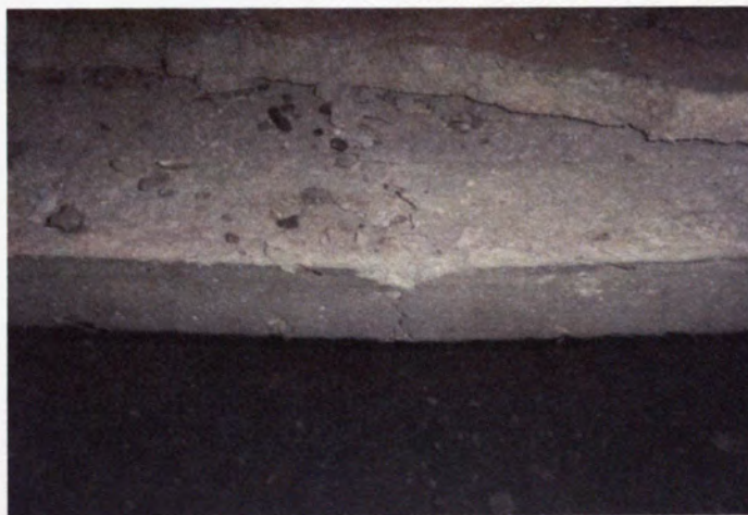
(e) Large Crack Back Face of Panel
