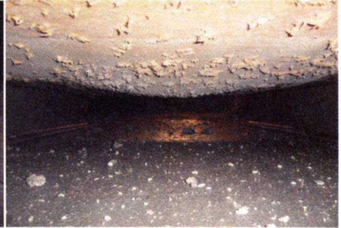
(f) Bulge in Tension Face
