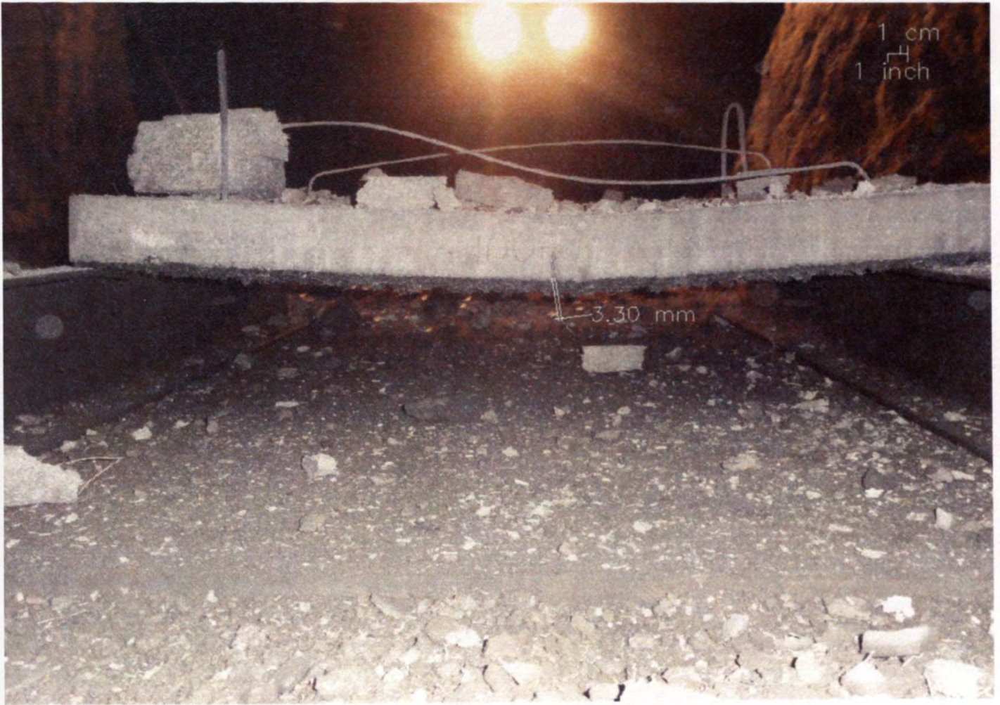
Figure E.13 – Flexural Cracks in the Back Face of H-FG-A/F, 2 nd Event
