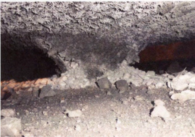
(e) Polyurea Tear and Rubble Tension Face
