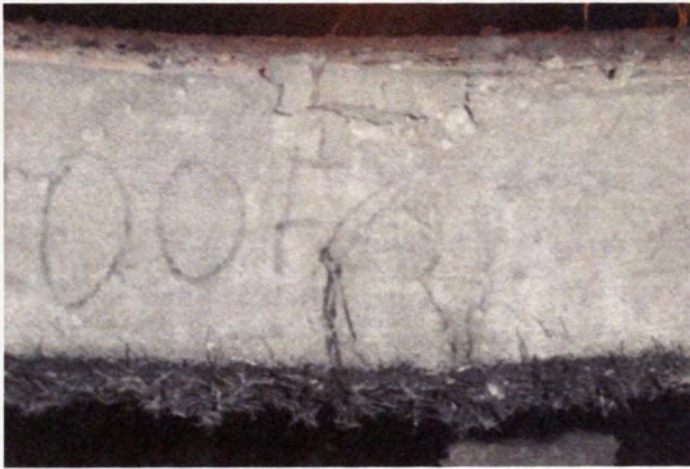
(c) Flexural Crack Back Face
