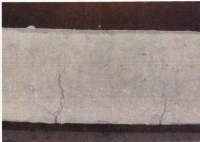
(c) Flexural Cracks on Back Face
