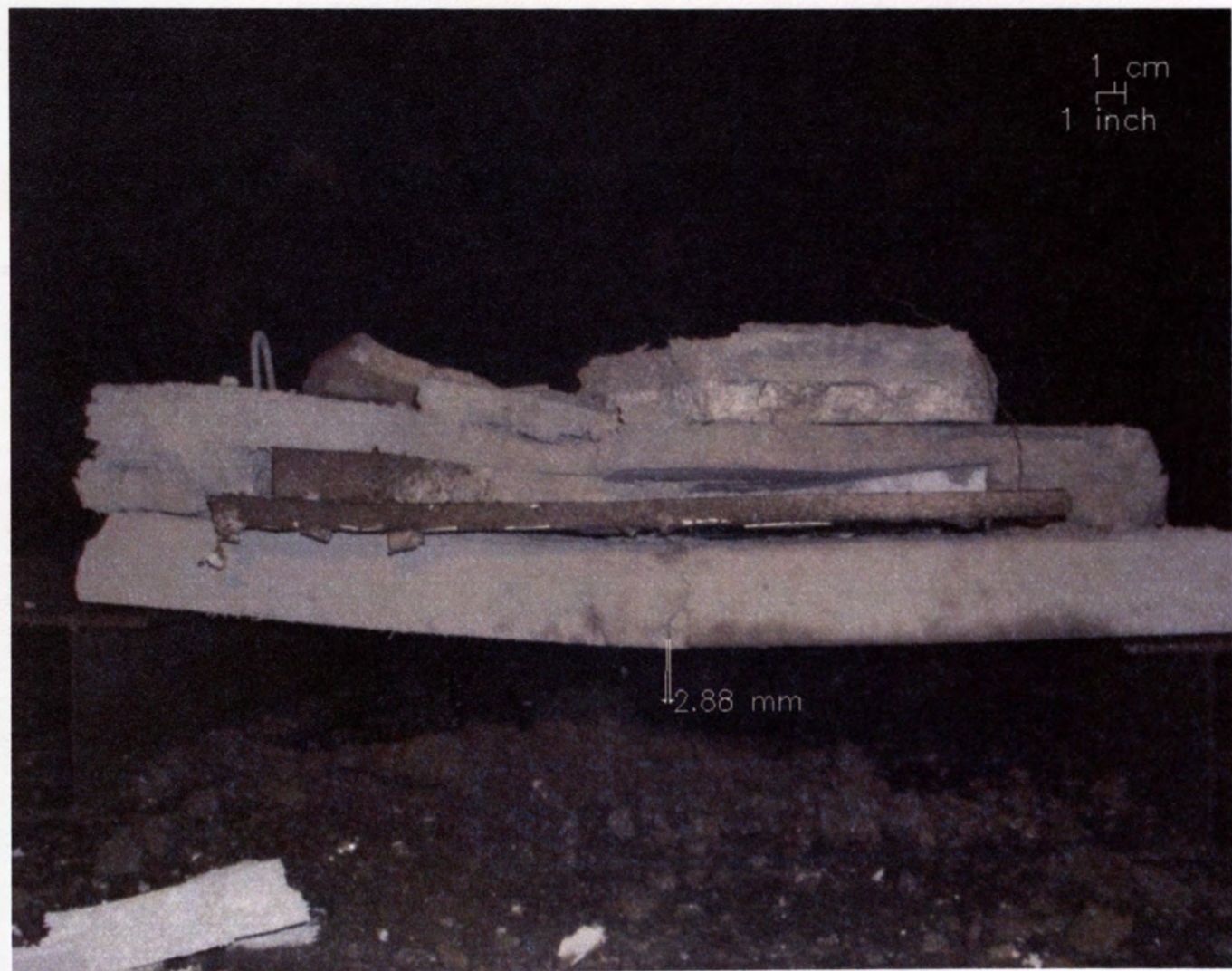
Figure E.10 – Flexural Cracks in the Front Face of H-FG, 2 nd Event
