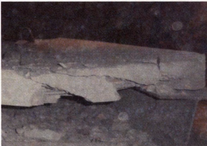
(c) Shear Crack in the Front Face
