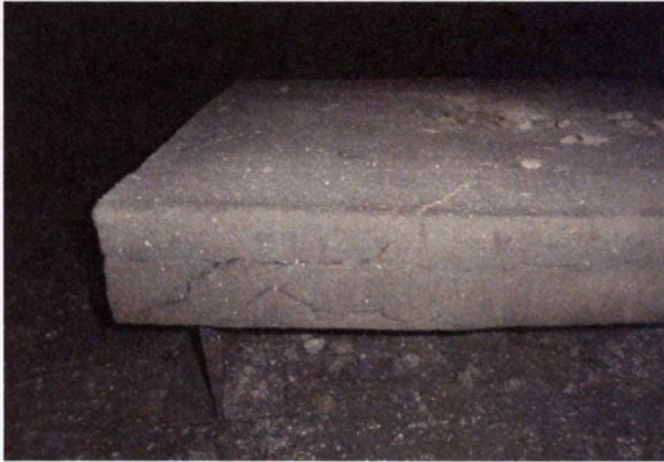
(c) Shear Cracking Front Face
