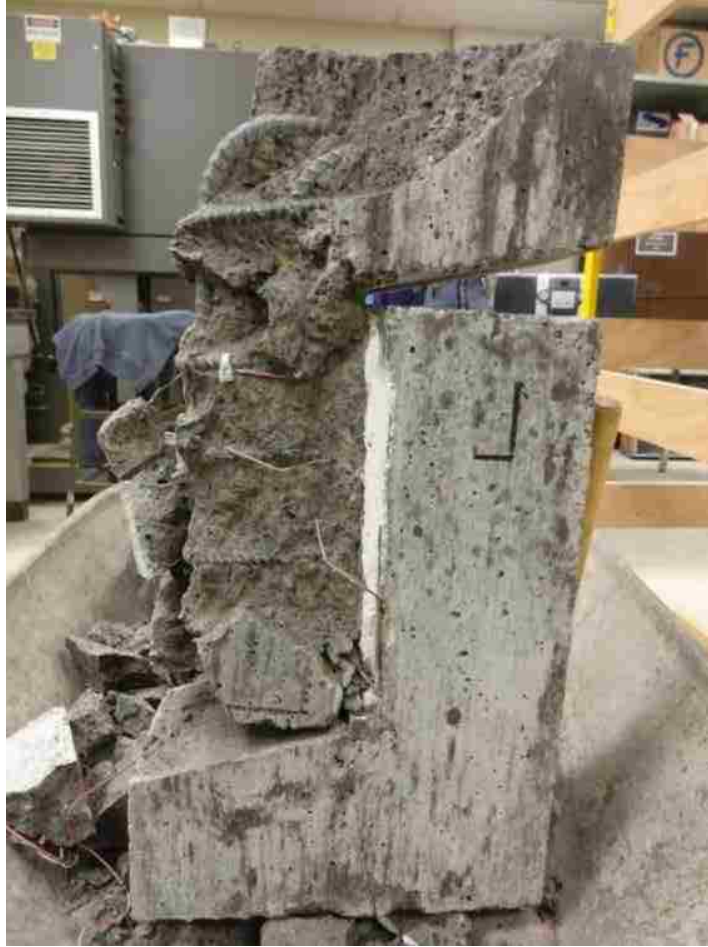
Figure 3.29. Specimen S-CL-CJ-R-17-2 with loose concrete removed, confirming that cracks extend to surface of longitudinal reinforcement bar (splitting failure)
