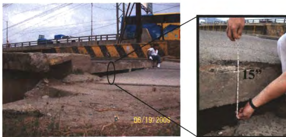
Figure 5-8: Differential Settlement at La Democracia Bridge on the Ulua River
