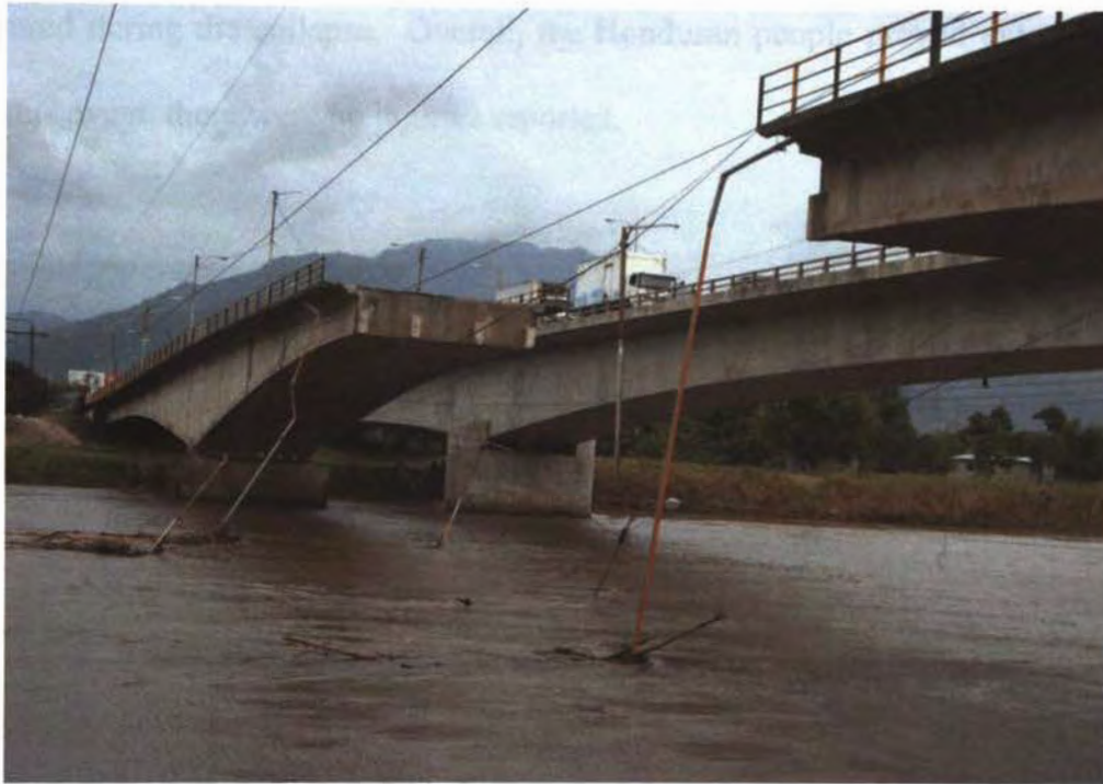
Figure 5-9: Collapsed Span of La Democracia and Surviving Sister Bridge
