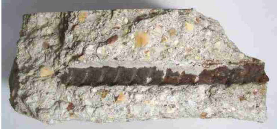
Figure 3.19: Red rust observed along the inner surface of a segment of 50/50 enamel that remained attached to a section of concrete.
