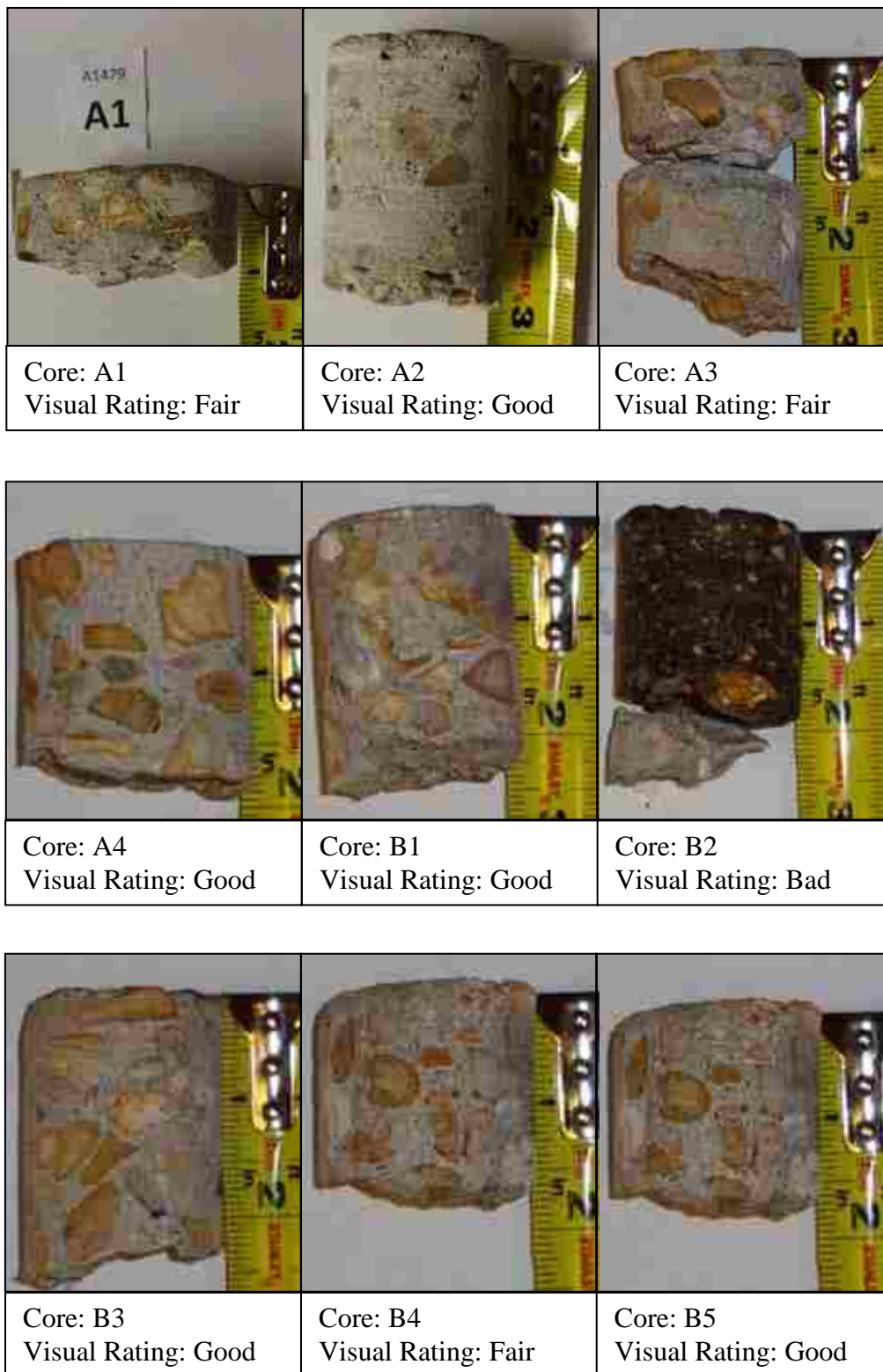
Figure 3.23. Bridge A1479 Cores and Visual Core Ratings
