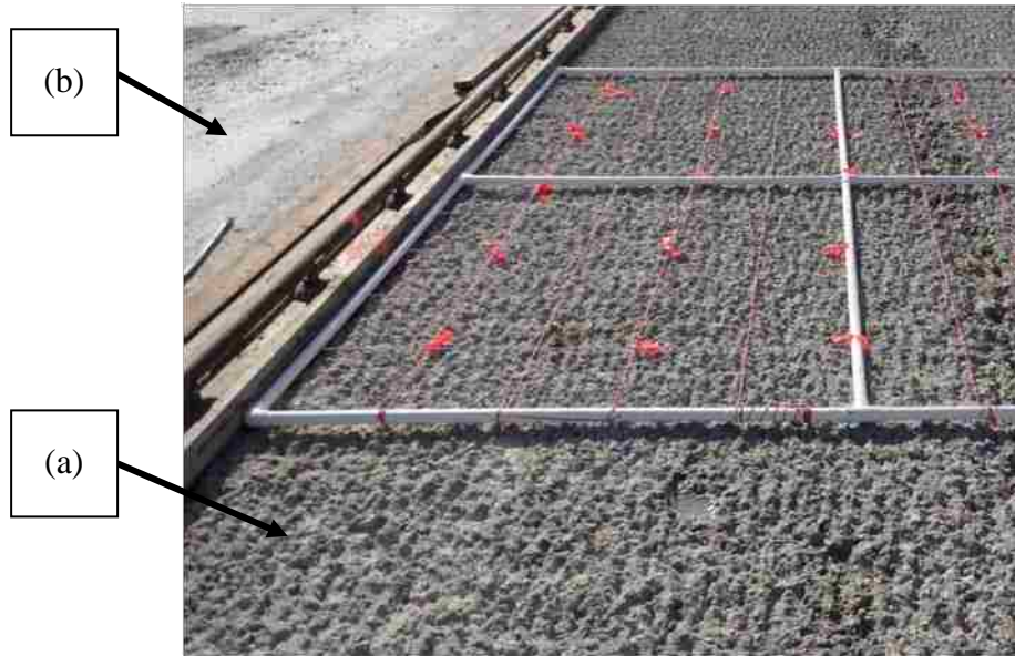
Figure 3.9. Rough Grooved Concrete Surface Caused by Milling (a) and Original As-Built Concrete Surface (b)
