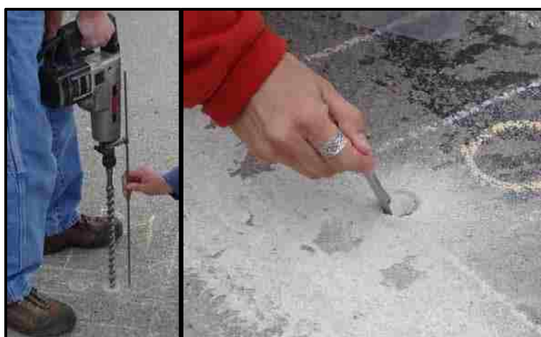
Figure 2.11. Pulverization Using a Rotary Hammer (Left) and Sample Extraction (Right) for Chloride Ion Determination
