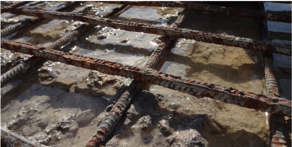
Figure 3.10. Corroded Rebar Exposed After Removal of Loose and Deteriorated Concrete by Hydrodemolition
