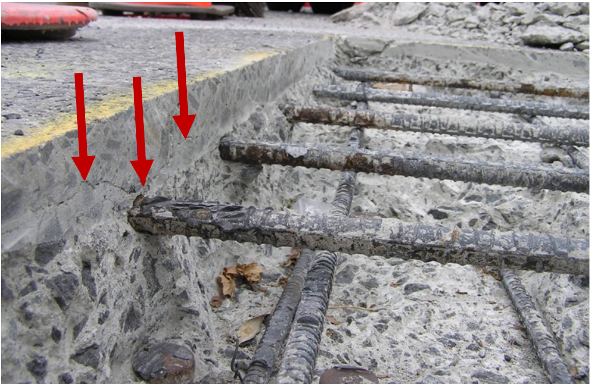
Figure 2.2. Delamination in Bridge Cross Section [6]
