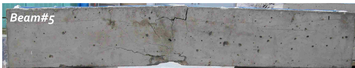
Figure A.4. Beam#5_ PC (mortar) _ Structural Epoxy
