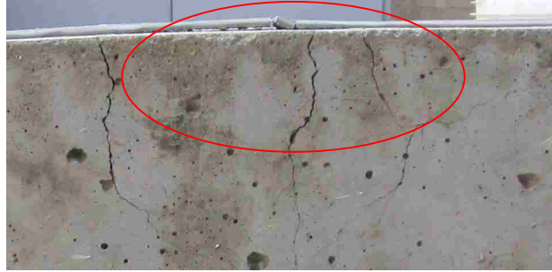
Figure 5.7 HoldTight 102 spalling at the midspan of Beam # 2
