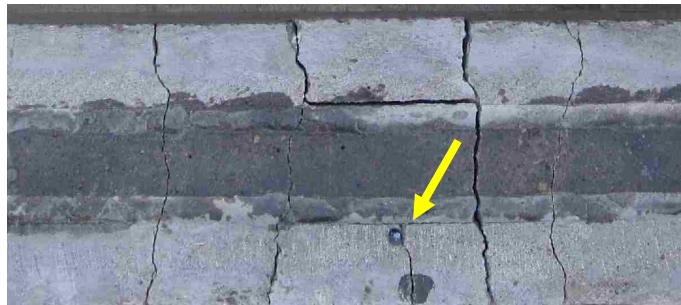
Figure 5.20. Close-up view of the crack pattern within the midspan of the tension face of the Beam # 6
