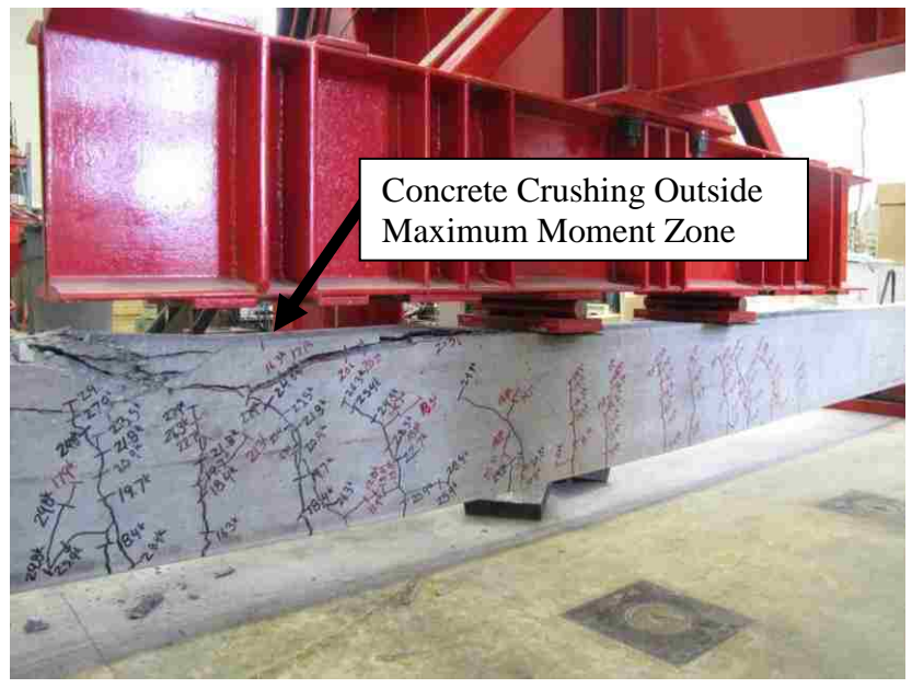
Figure F.15 – S6-2-2_73 at Failure
