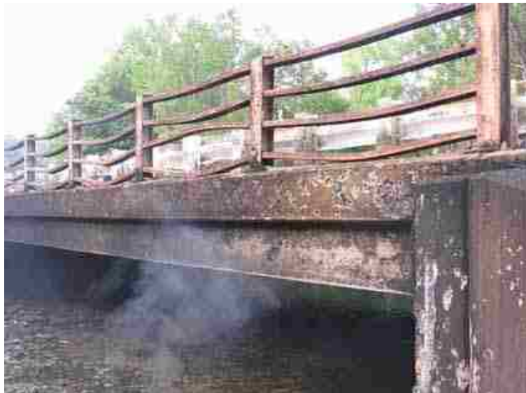
Figure 2.7 Damaged Norwalk Bridge near Ridgefield, Connecticut due to an overturned gasoline tanker (FHWA, 2007)
