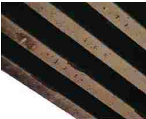
Figure 6.8 Damaged concrete located at the bottom of the girders (location which was closet to heat source) (Aspire, Spring 2008)
