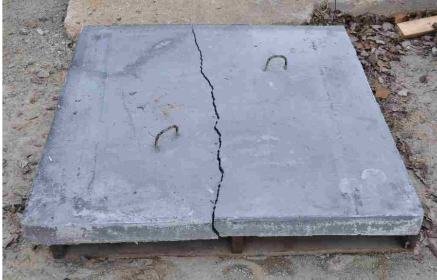
Figure 6.29. Broken 3.5-in plain UHPC panel
