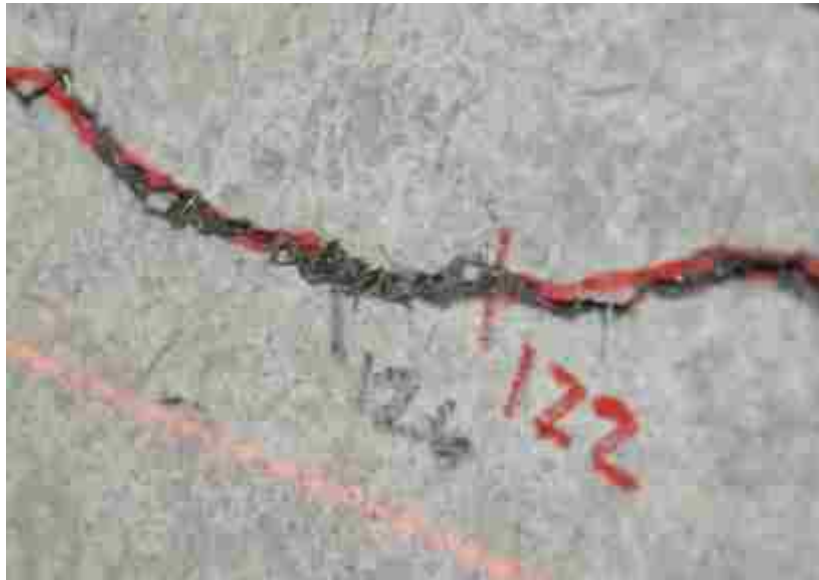
Figure 6.12. Fibers bridging bottom crack of I-2-6F-2
