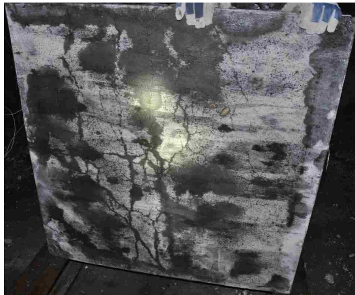
Figure 6.19. Bottom face of B-3-2F-3.5 after detonation
