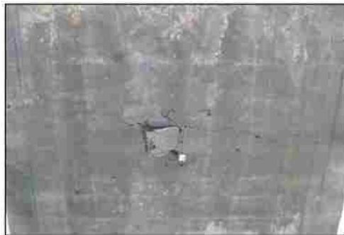
Panel 3 rear surface after explosion - Very slight scabbing at surface of the panel - Minor cracks through panel. - Structurally undamaged.
