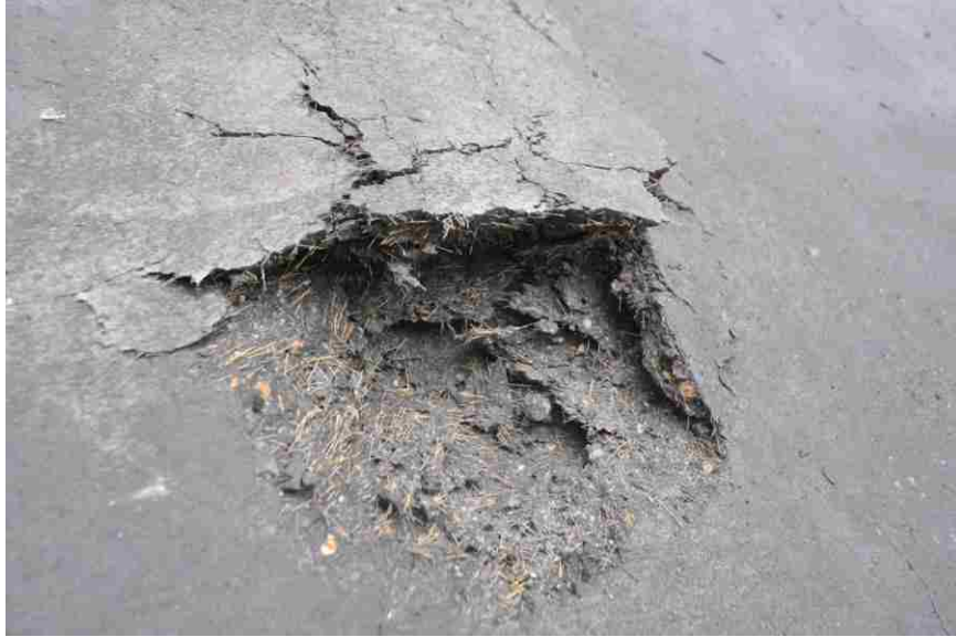
Figure 6.52. Close-up of spalling on H-3-6F-3.5
