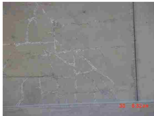
Figure 2.2: Cracking observed in partial-depth precast-prestressed concrete panels in Colorado (Courtesy of Colorado DOT)
