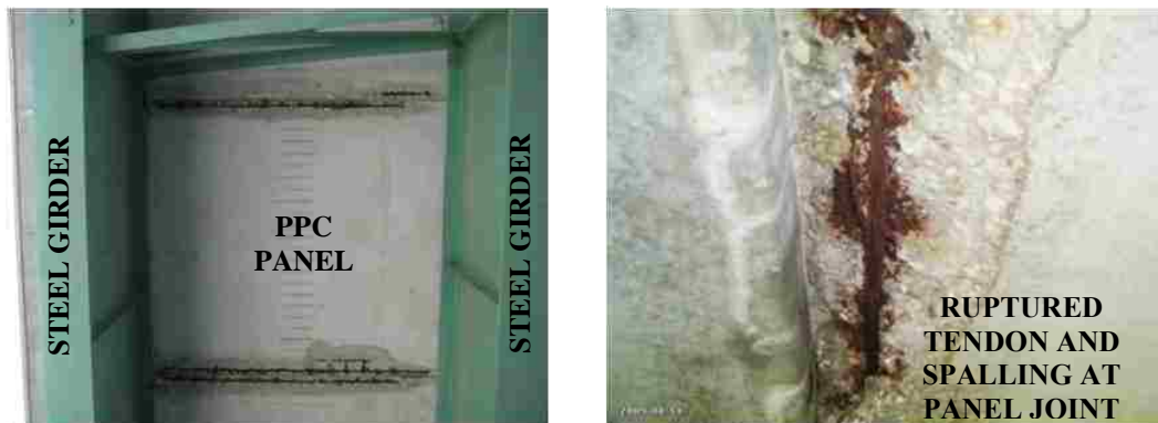
Figure 1.2: Spalled sections of concrete at various panel joints
