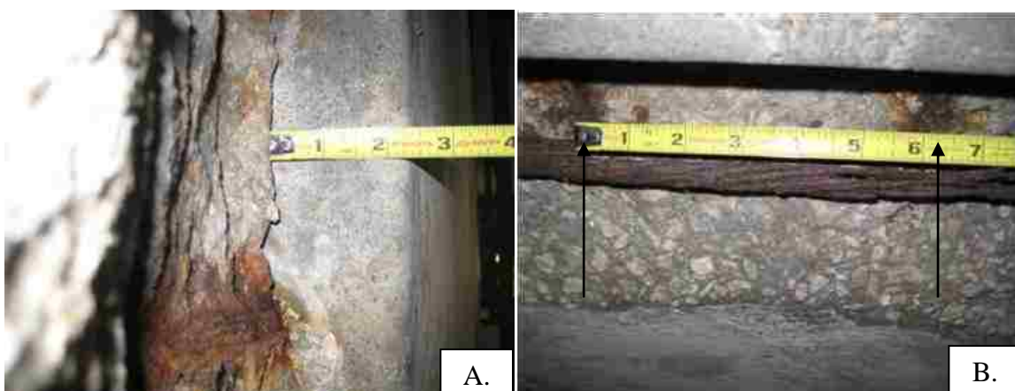
Figure 3.4: Spalled sections of PPC panels (A. Depth of a spalled section, B. Exposed mild reinforcement in a spalled section) (Bridge A4067)
