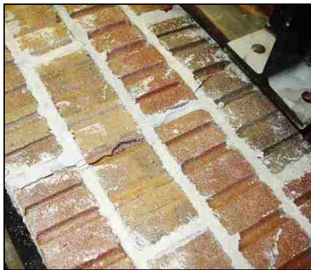
(a) Longitudinal Cracking
