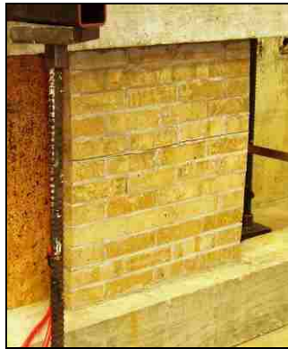
(a) Horizontal Cracking
