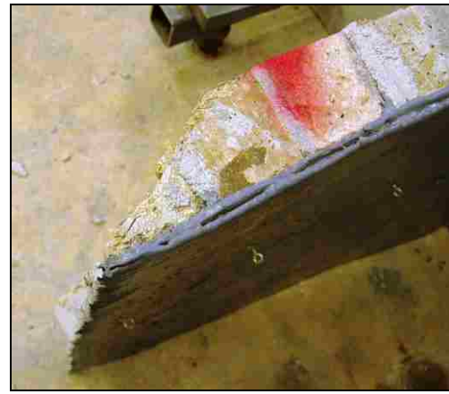
(b) Damage Sustained to WF-FA Units
