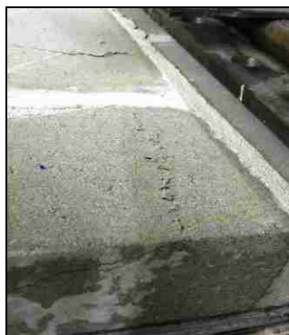
(a) Flexural-Shear Cracks
