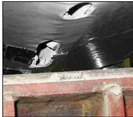
(c) Rupture of Polyurea
