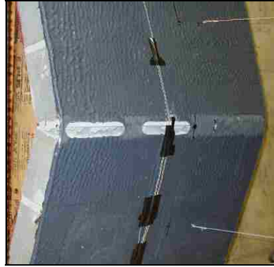
(b) Rupture of Polyurea
