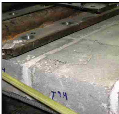
(a) Masonry Rupture
