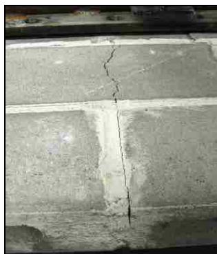
(b) Longitudinal Cracking
