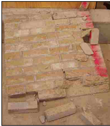
(a) Wall Collapse
