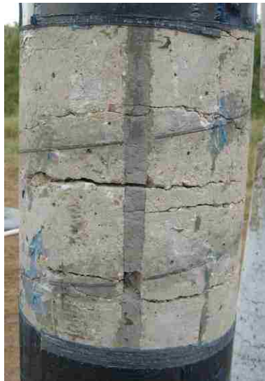
Figure 6.16. Back Side of Column 3
