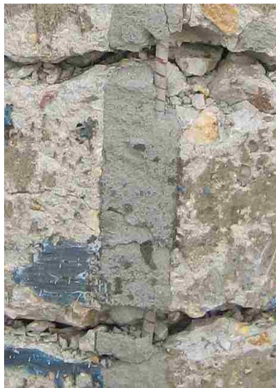
Figure 2.5. Separation of Steel Spirals in Two Cracks
