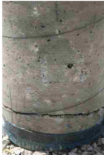
(a) Crack at Base
