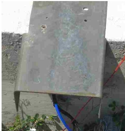
Figure 5.5. Steel Plate to Protect Sensor Connectors
