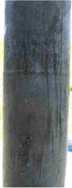
Figure 6.11. Damage to Front Side of Column 3 after 10 lbs Blast
