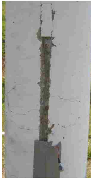
Figure 6.2. Damage to Sensor Grout on Column 1 after 1 st 4 lbs Blast
