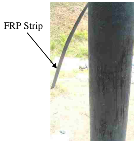
Figure 6.8. Damage to Column 3 after 2 nd 4 lbs Blast
