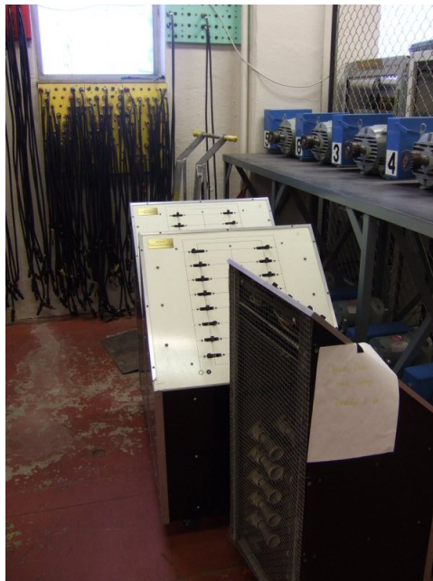
Figure 5.9: The static load banks.
