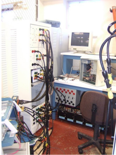
Figure 5.8: The programmable load bank console.
