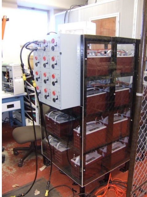
Figure 5.10: The load bank power storage array.
