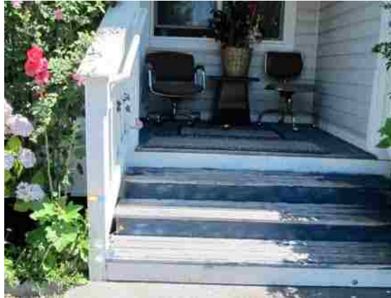
Image 22: First Two SHA-Rental Units' Porch and Stair Material Wearing and Deteriorating Compared to a Market-Rate Unit's Porch and Stair Materials with Better Quality (Third Photograph)
