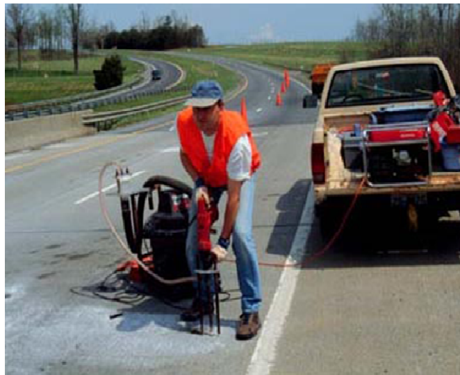
Figure 2.7. Sampling for chloride concentrations – collection apparatus: impact drill with hollow drill bit, powder concrete collection unit, and vacuum (Zemajtis 1998)
