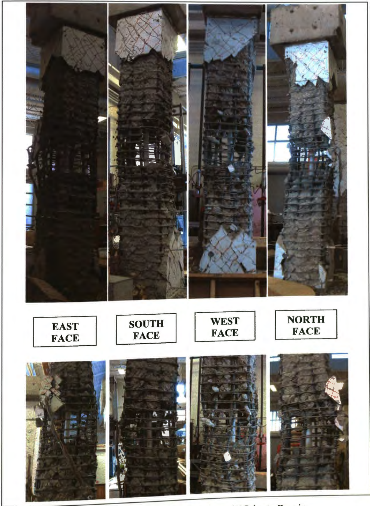
Figure A-6. Damage Photos of Column #6 Prior to Repair
