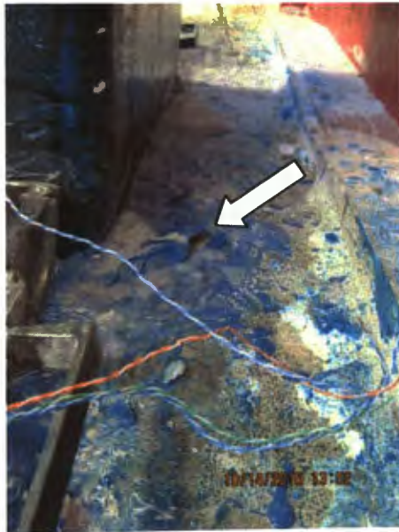
Figure 5.4. Pullout Failure of U-Anchors for Column #2
