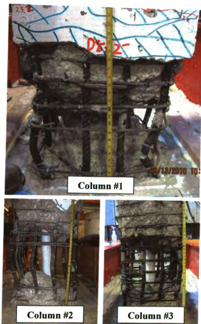
Figure 4.16. Columns After Removal of Loose Concrete
