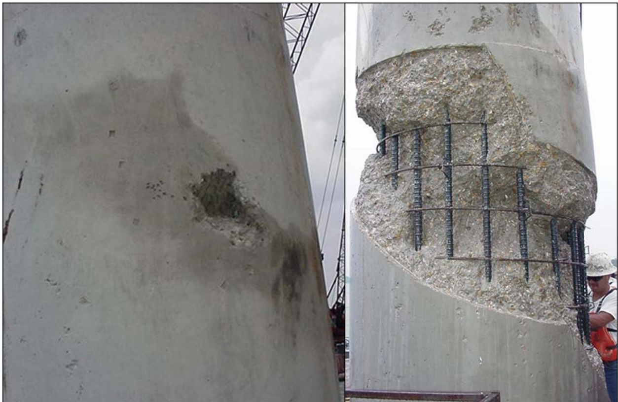
Figure 3.1 Soft concrete visually identified (left); full anomalous extent removed (right).
