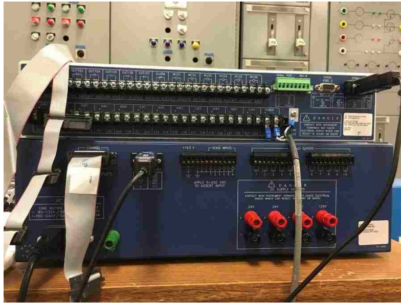
Figure B.1. Image showing connections of SEL AMS to SEL 387 relay
