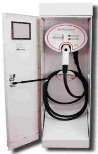
Figure 2.12. An image of the EV charge station in the solar village.
