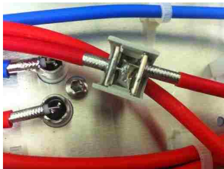
Figure 2.30. Potential PIM source location I: Solder joint.
