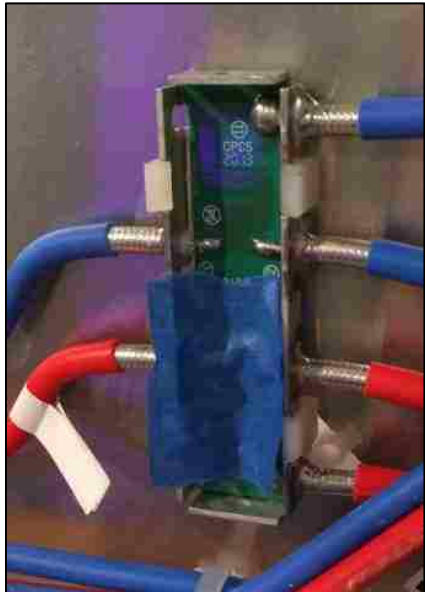
Figure 4.3. Ferrite debris as PIM source on power divider.
