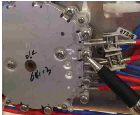
Figure 4.6. Loose screw on the phase shifter as PIM source (indicated by the tip of a pen).
