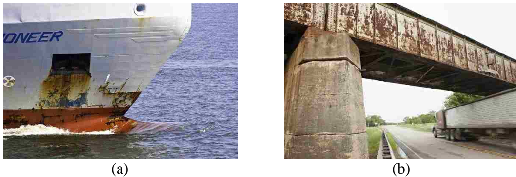
Figure 1.1: Photos of two severe corrosion cases on painted steel: (a) on an aquatic vessel (source: www.futurecleansystems.com ) (b) on a steel railway bridge (source: www.mprnews.org ).
