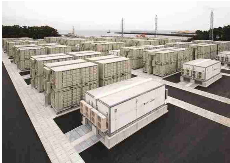
Figure 1.10. Stationary battery units. Courtesy: Mitsubishi Electric [30]
