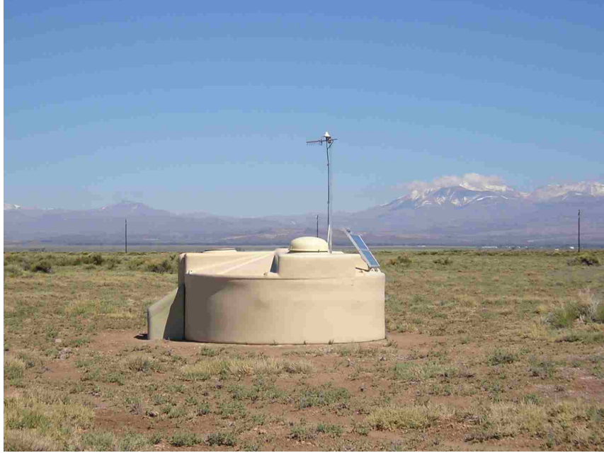
Figure 2.2: A working SD station. The communication antenna and solar panel to charge the batteries are visible.
