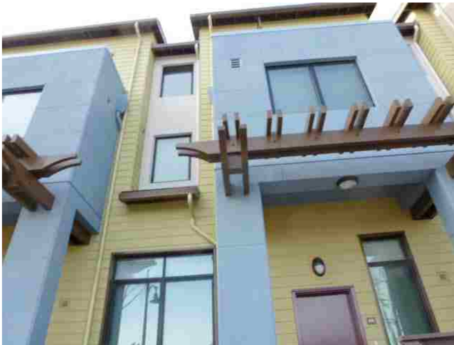
Image 46: Close-up Photo of Phase VI Building with Saturated Paint Color
