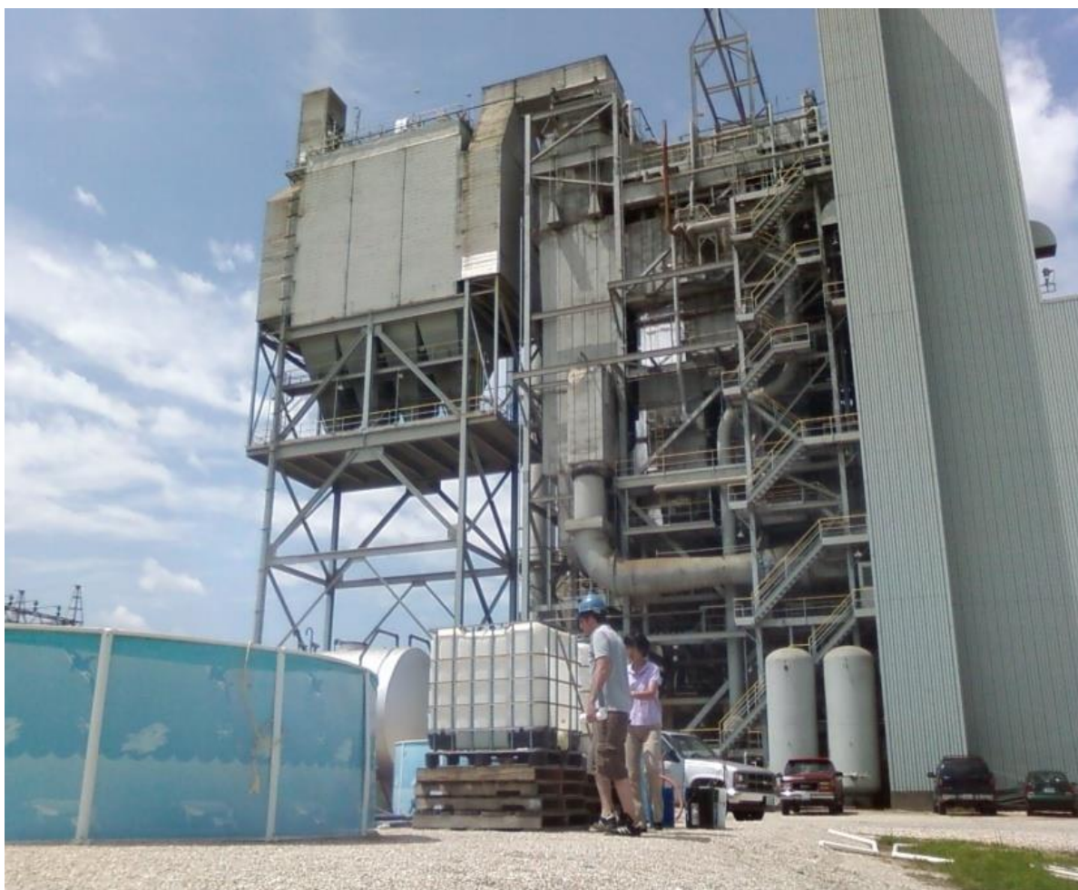
Figure 1. Coal fired power plant, Central Electric Cooperative power plant Chamois, MO.
