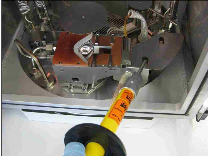
Figure C11 Probe touching high voltage conductor.
