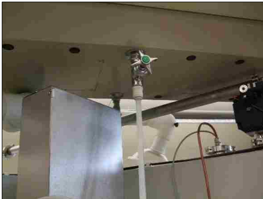
Figure C3 Location of the cooling water source.
