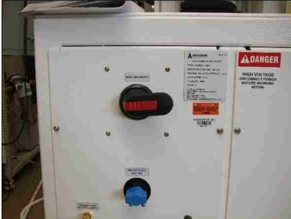
Figure C4 Location of the main disconnect.
