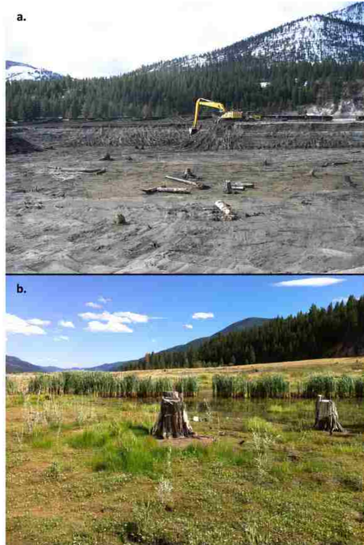
Figure 4.2. (a) During remediation, excavation activities uncovered numerous trees beneath the former reservoir’s surface, indicating where the historical floodplain previously resided. Trees identified included cottonwoods and ponderosa pine. (b) Over 600 relict tree stumps populate the lower portion of the restoration area today. Tree diameters range from <20 cm to > 1m.
