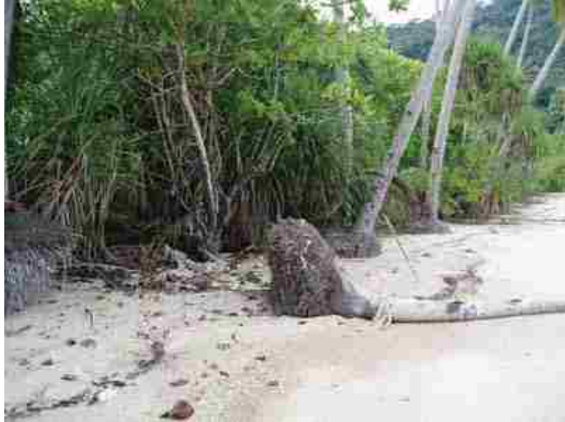
Figure 7.8: Exposed tree roots and downed trees due to sand erosion
