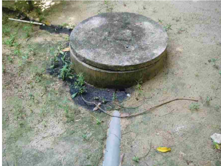
Figure 7.9: Leaking septic system
