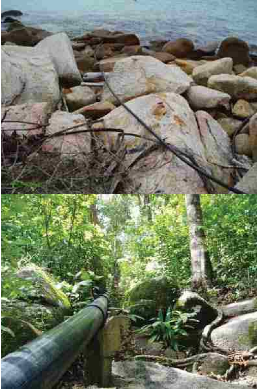
Figure 4.9: Electricity and water supply lines crossing tourist areas.
