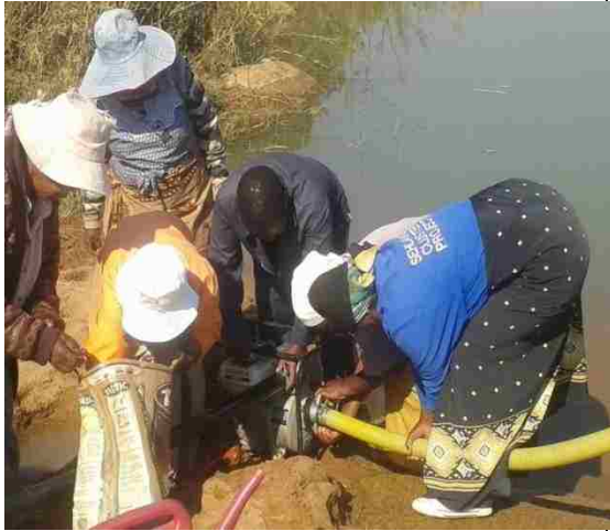
Participants busy connecting a hosepipe to the generator to pump water from the river to the garden.
