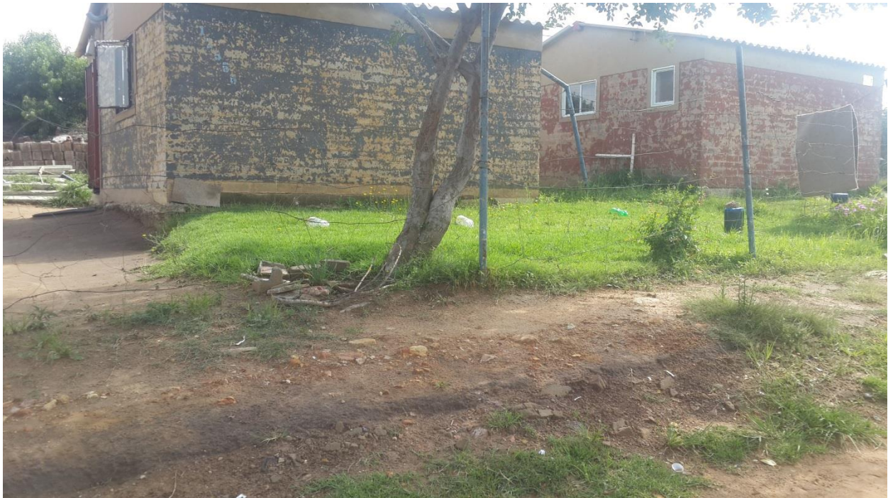
Fig. 5.3 Plastering flaking off due to poor building materials used: Photos by JM Kotane
