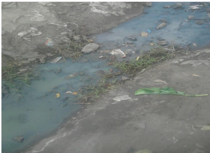
Plate 7. Blocked drainage at Mandevu market in Lusaka City
