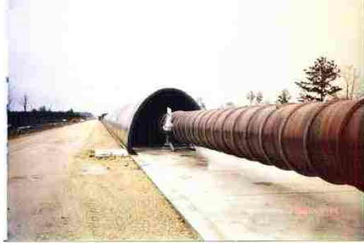
Figure 6-7: A picture of LIGO Livingston’s beam tubes during construction. Photograph credit: Larry Jones (c1998).
