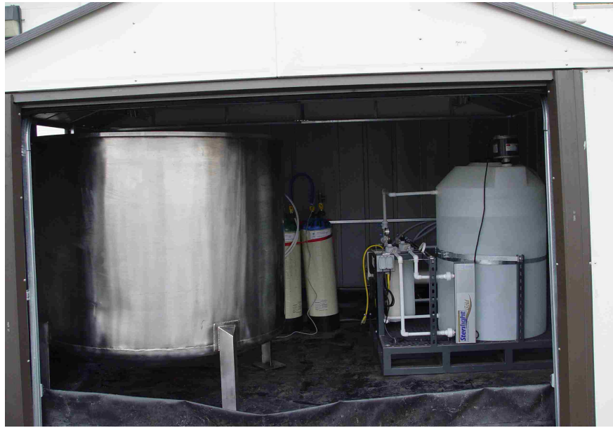
Figure 4.5: The water hut with the front sliding door in the open position. The purification system, test tank, and portable resin beds all sit inside a secondary containment berm.
