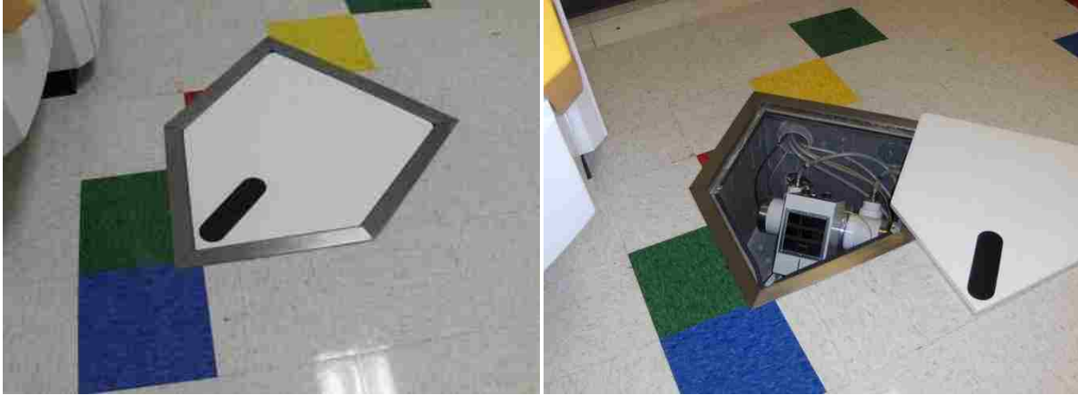
Figure 3.5: Picture of covered kV x-ray housing panel in floor (left) and with cover removed (right)
