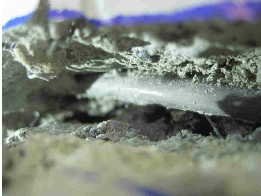
Figure C - 4: Large crack in concrete core, cycle 9-1.
