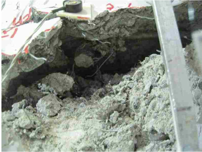
Figure 4-8: PreT-BS broken longitudinal rebar.
