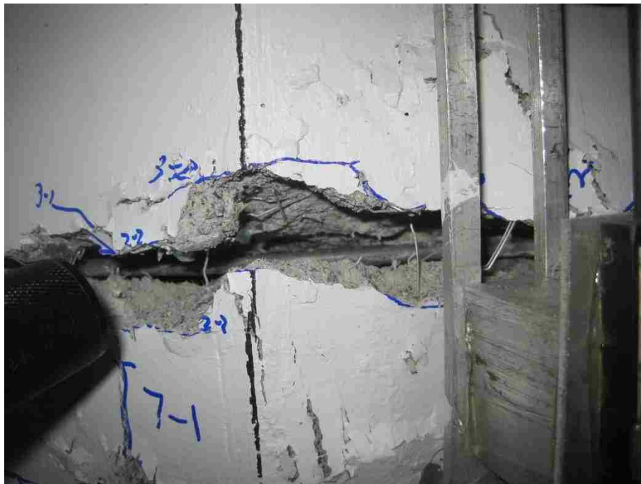
Figure C - 11: Large crack in concrete core, cycle 8-2.
