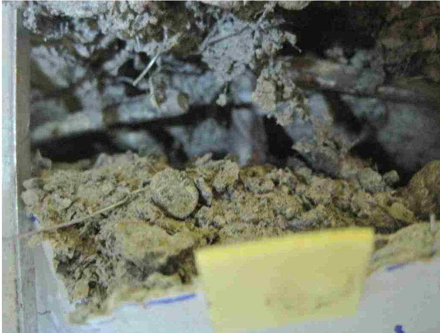
Figure C - 12: Fracture of longitudinal reinforcement bar, cycle 9-2.
