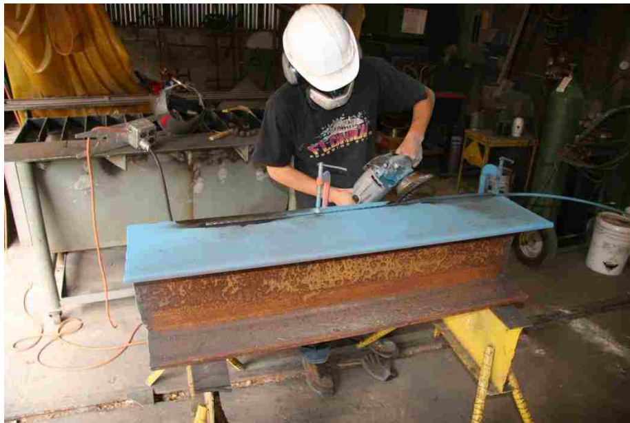
Figure 2-12: Strands prepared for stressing. Epoxy coating taken off so chucks can grip safely to strand.
