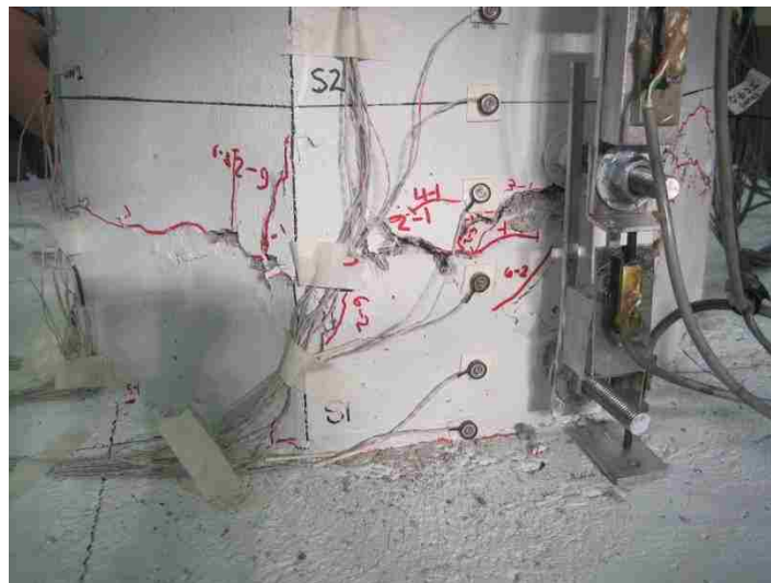
Figure 4-4: PreT-BS significant spalling in column during Cycle 7-1.
