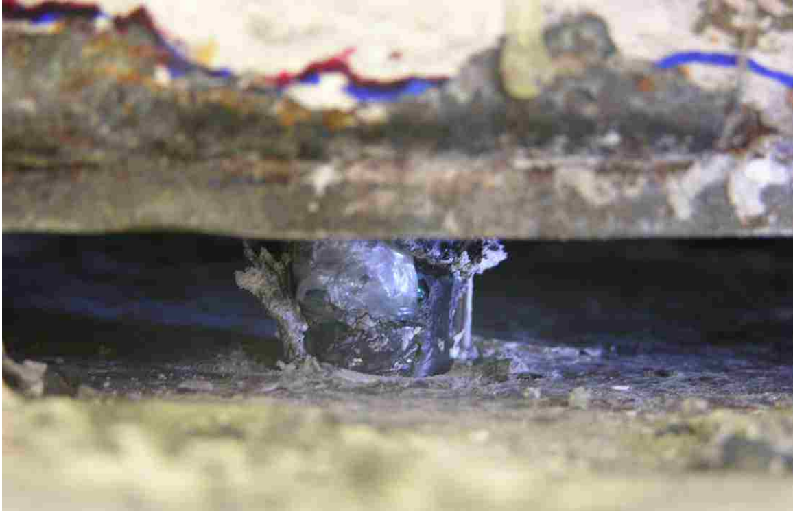
Figure C.11 Exposure of rebar.
