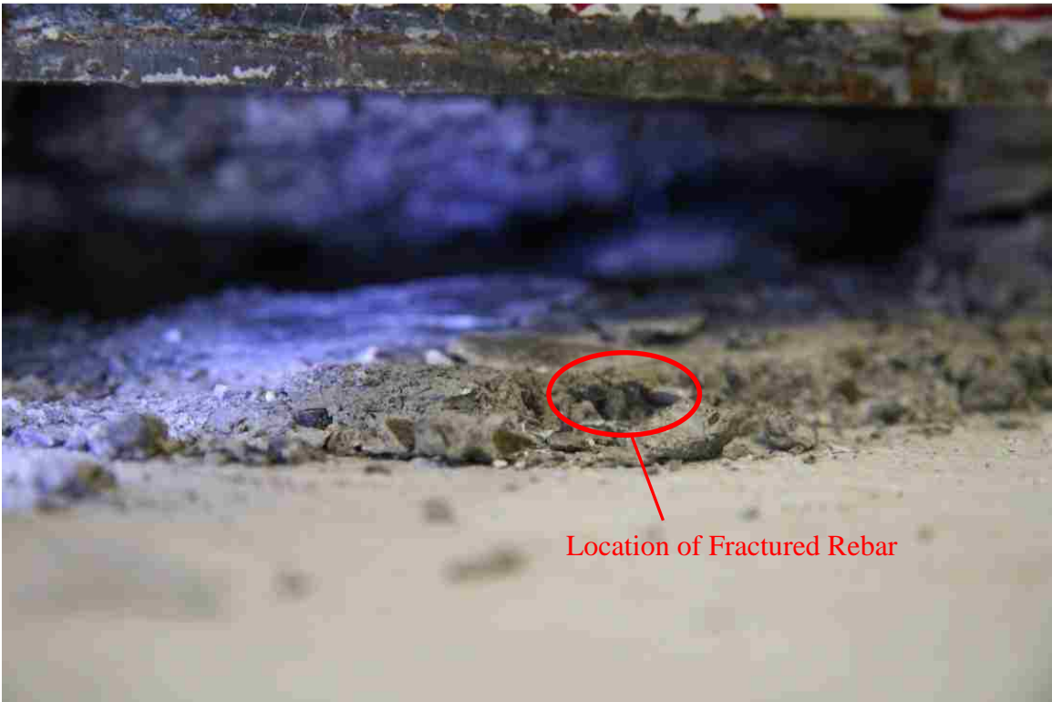
Figure C.3 Fractured Rebar, cycle 9-1.
