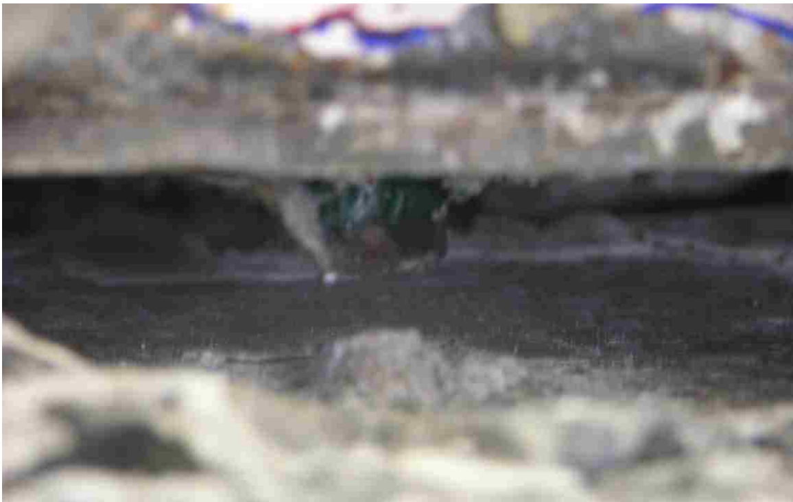
Figure C.12 Fracture of rebar.
