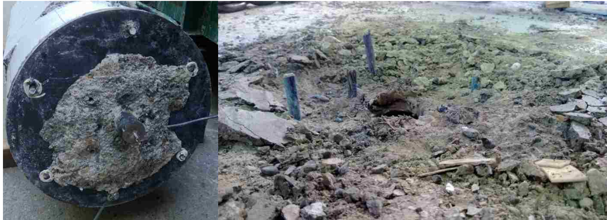
Figure 4.8 Jagged portion of HyFRC that seeped through steel-wire mesh (Left). Column-footing interface after top portion of column was removed (Right).
