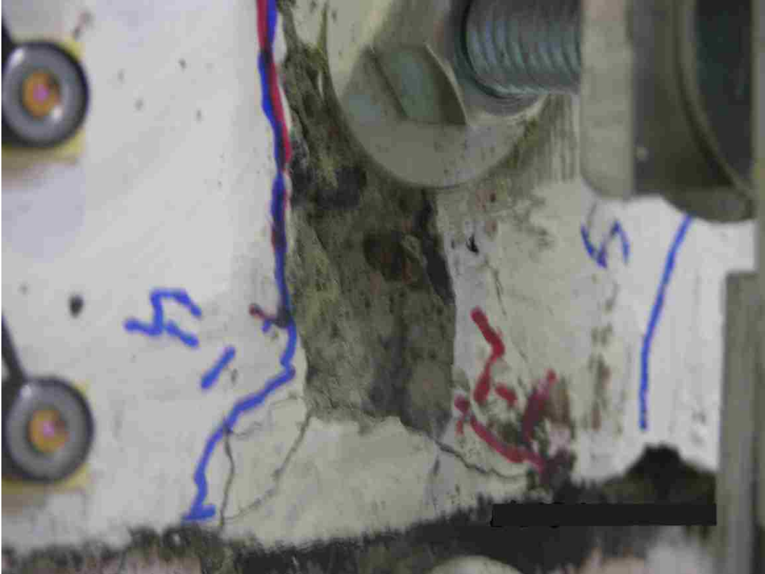
Figure C.9 Cosmetic spalling at top of shoe.
