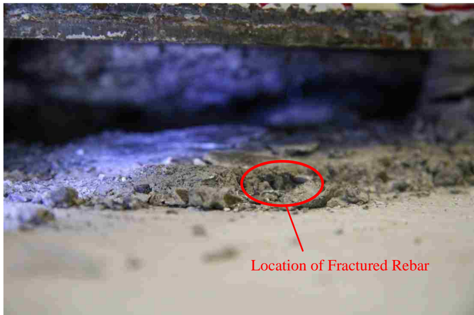
Figure 4.10 Fractured northwest bar of PreT-SF-ROCK-HyFRC (fractured in footing).
