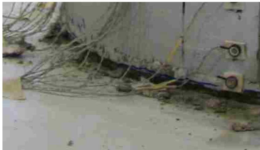
Figure 4.7 South view of PreT-SF-ROCK-HyFRC showing the fillet spalling of the footing induced by the rocking action of the steel shoe.
