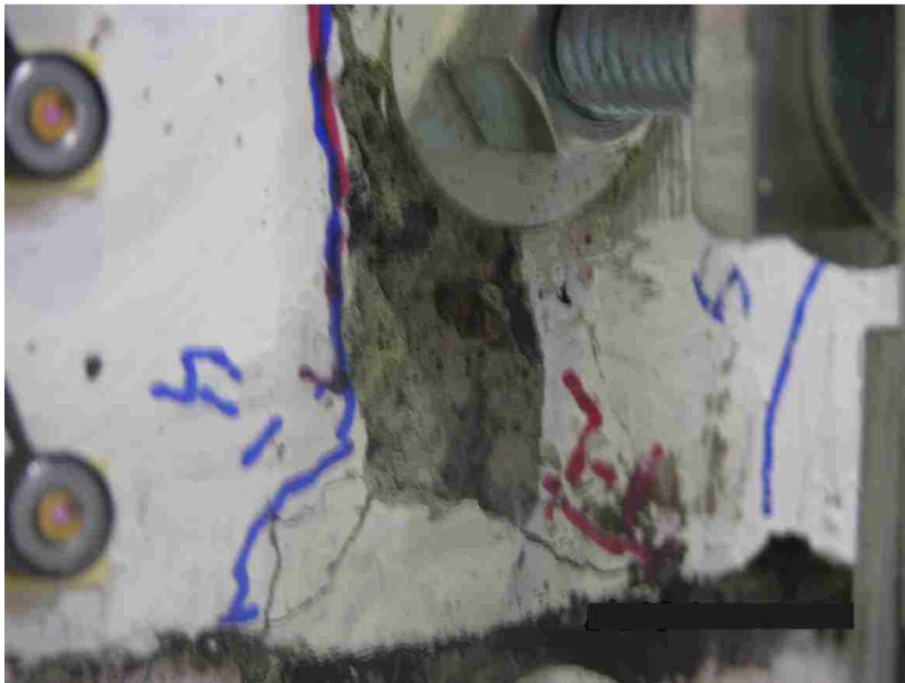
Figure 4.5 South view of PreT-SF-ROCK after cycle 8-4 showing spalling damage above the steel shoe.
