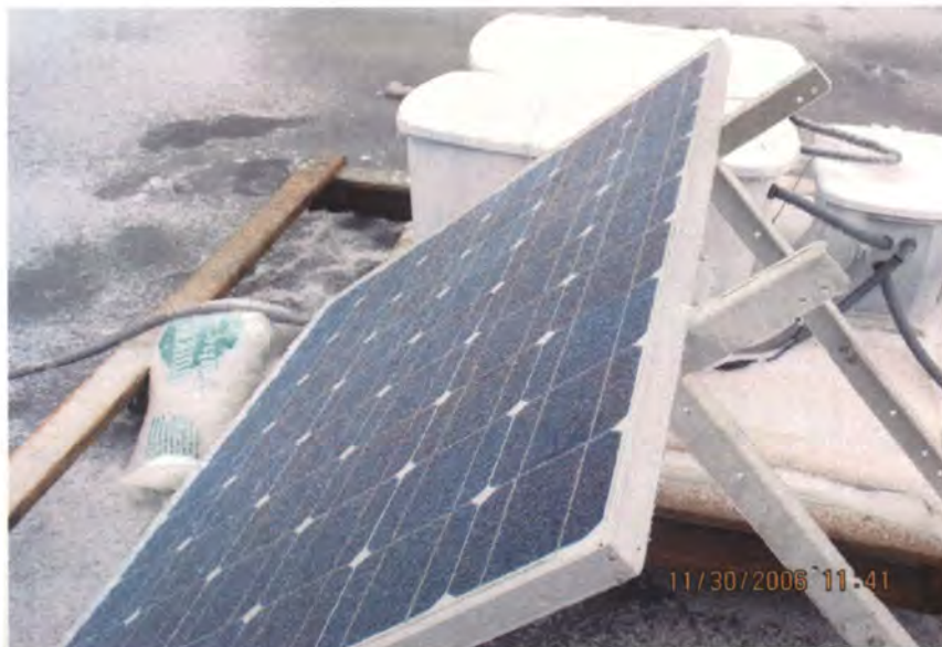
Figure 2.5. Panel Covered in Ice at the Start of the Storm
