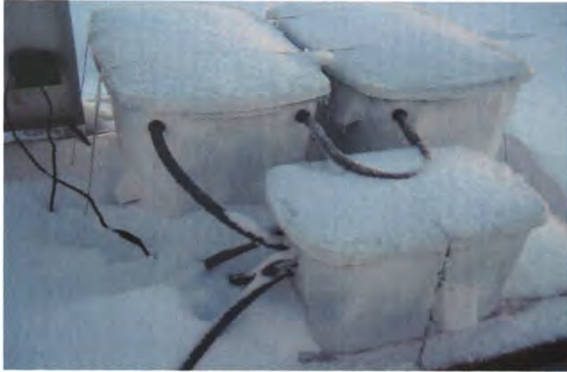
Figure 2.7. Two-Inch-Thick Ice on the Battery and the Controller Containers
