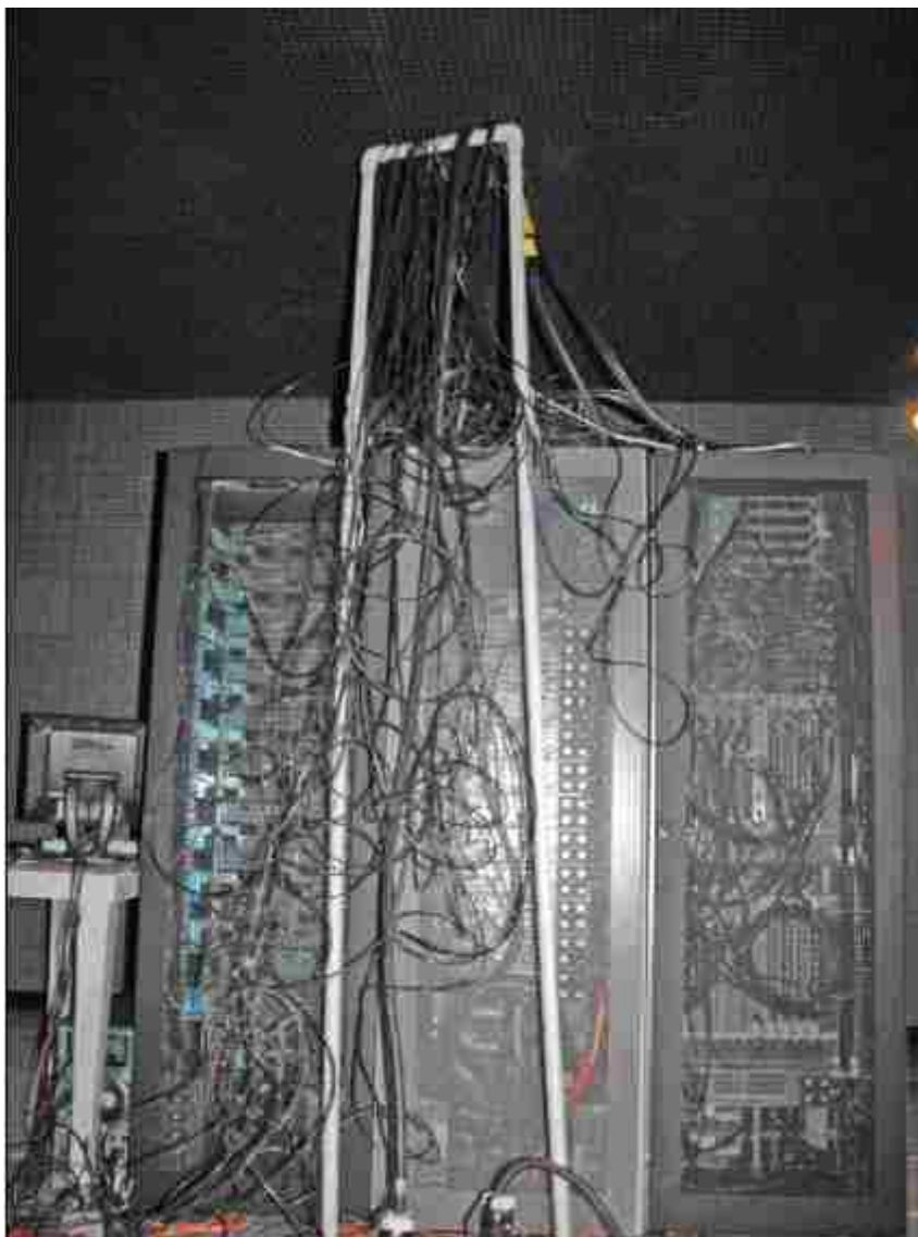
Figure 1.13. Cabinet Rack with the Cable Harness Egressing From the Top
