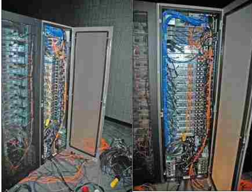
Figure 1.2. Digital Photographs of the NCR Node Rack Equipment from Two Different Angles
