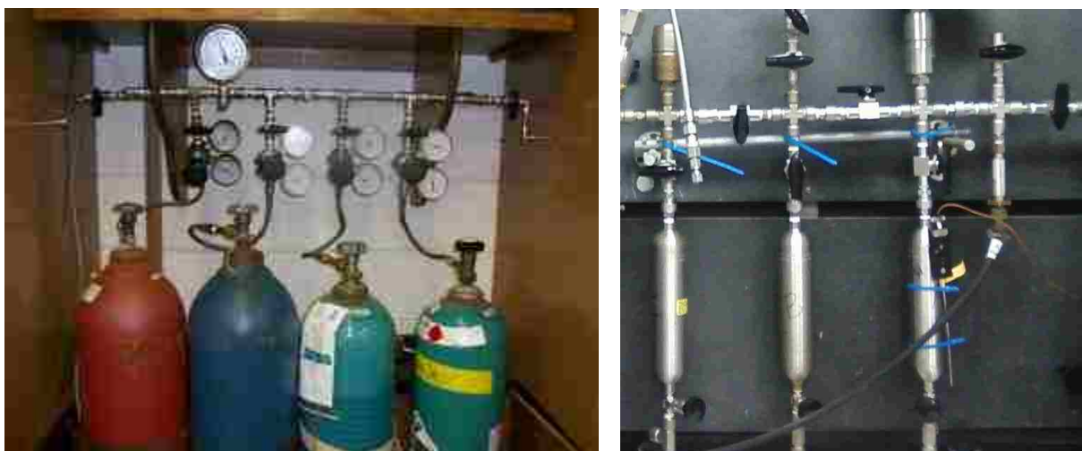
Figure 3.4. New/current gas manifold system. Source gas cylinders (left) and the manifold gas reservoirs supplying gas to the autoclave (right).
