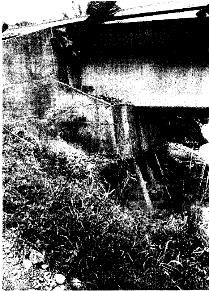
(a) Abutment failure at Rio Banano bridge, Costa Rica earthquake 1990
